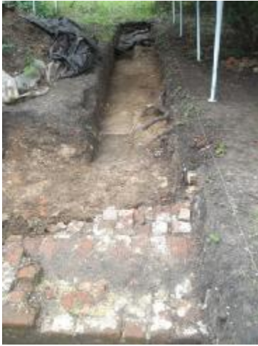
The trench containing the foundations running West-East in the North-East wing, near the standing pillar.
